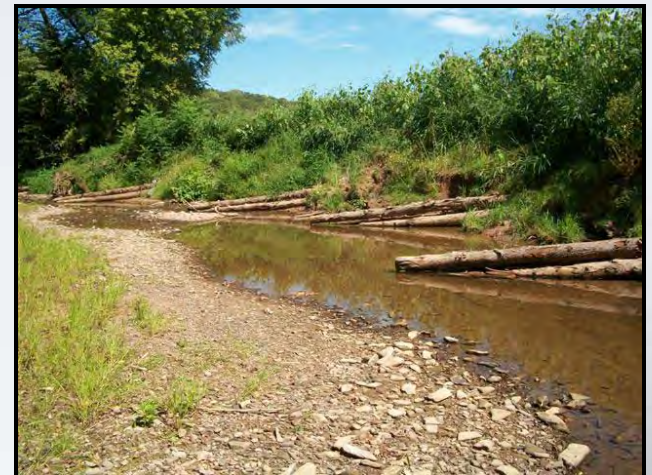
Log veins placed for streambank stabilization on the Tim Landis property in Herndon
