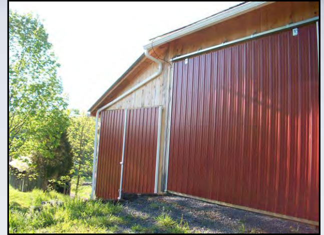
Installation of roof gutters on the Tom Rebeck farm in Dornsife, May 2010
