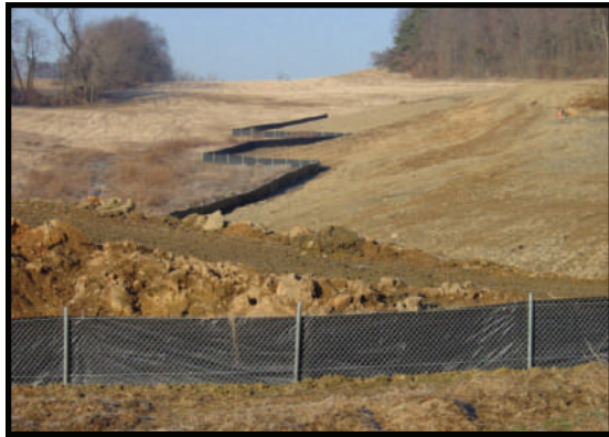
This is a silt fence used to eliminate sediment from eroding from a construction site.
