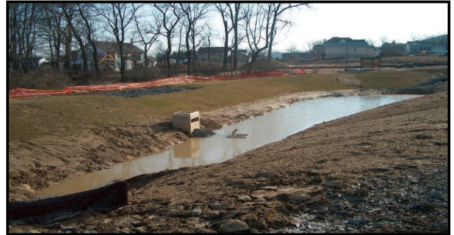
A sediment basin is just one of the many practices which can be utilized to help minimize the impact construction activities can have on our local waterways.
