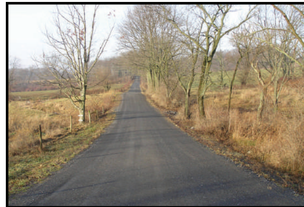
Here is a picture of a completed Dirt and Gravel Roads project on Swank Road in Rockefeller Township
